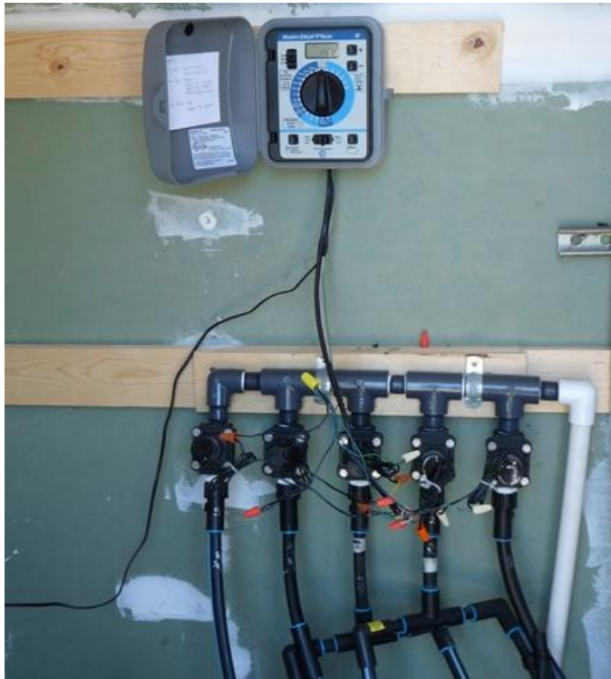
A fully automatic system to water a large yard
